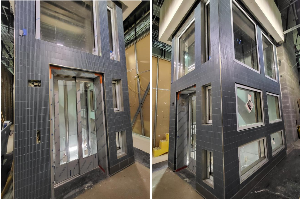
New second elevator
